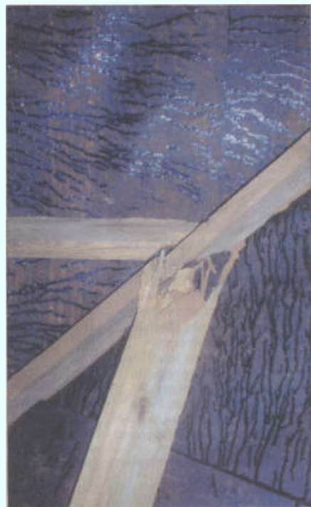
Dangerous: Although termites can cause
